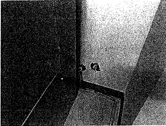
Photo 5 – Hole in Wall to be Sealed
