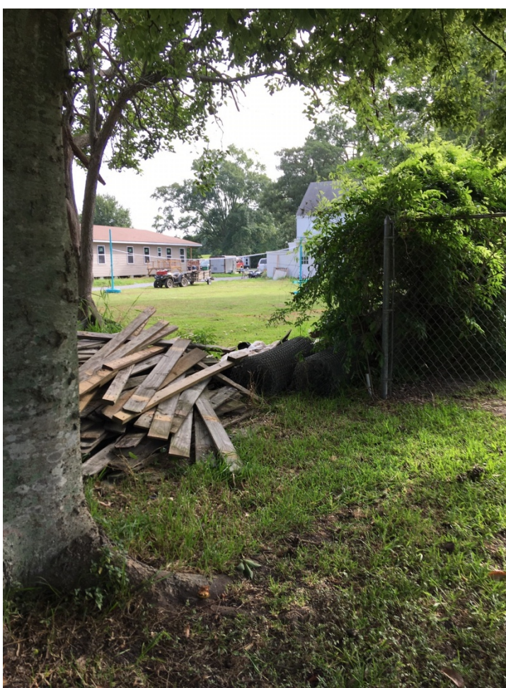
This picture shows more debris from a newly constructed wooden fence. When they were spreading loads of dirt to level the property, the Bobcat destroyed the fences on both sides of the property. They subsequently tore down the remaining fence that was still standing and deposited it against Mr. Hymel's fence. Some of the boards are actually encroaching on my property.
