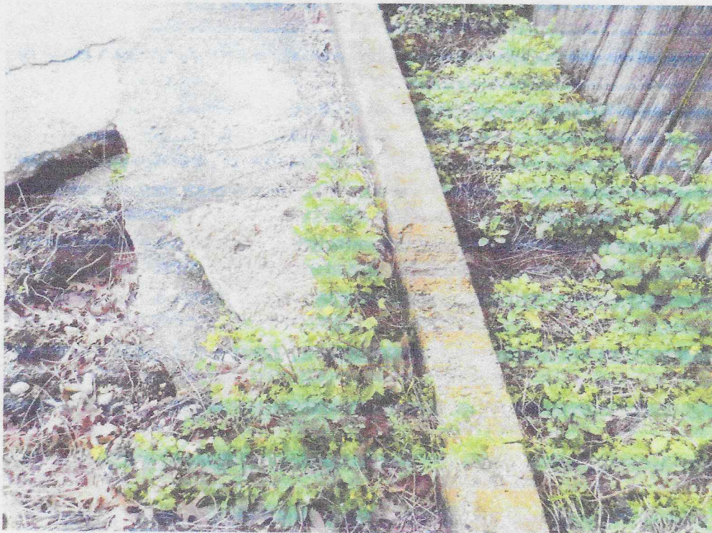
Figure 2. Damage to parking lot from pond on Civet property.
