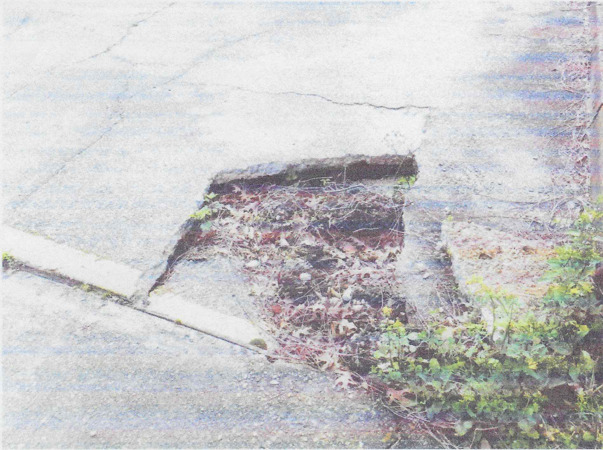
Figure 3. Photograph of the undermining of parking lot and loss of parking spaces due to siltation of swale and formation of pond that directs flooding to houses on Houmas Place. This is a violation of Parish Ordinance 25-35(a).
