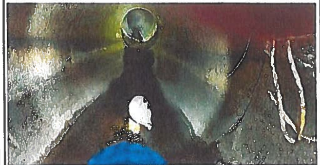
Exploratory Excavation @ Sta. 121+00. Existing DL looking from outfall at the Canal side.
