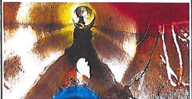
Exploratory Excavation @ Sta. 121+00. Existing DL looking from outfall at the Canal side.
